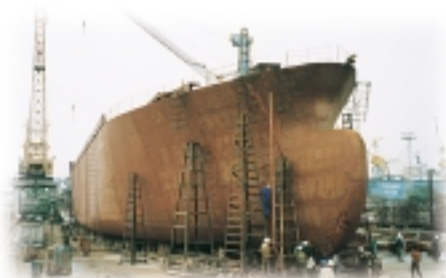
A 6,500 dwt dry cargo carrier being constructed in Vietnam by Bach Dang Shipyard
